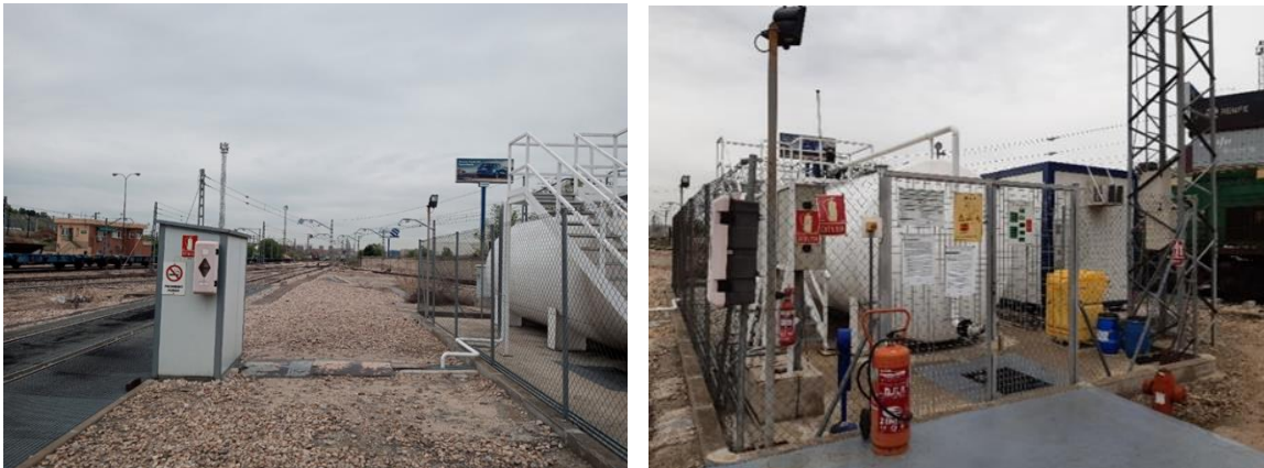
Figure 36: Diesel refuelling facility (example). Source: ADIF
