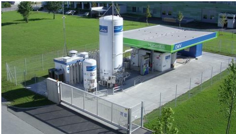
Figure 7: Liquid hydrogen refuelling station [9]
